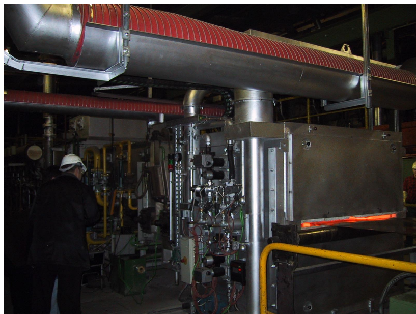
Figure 6: FLOX ® nozzle field in operation
